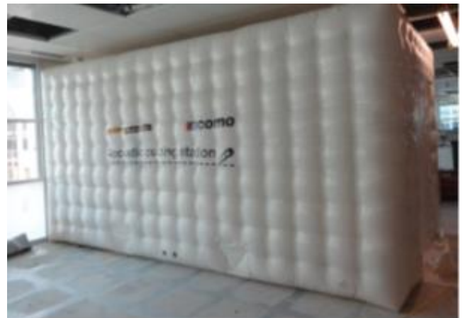
Figure 1: Inflatable acoustic cutting station
