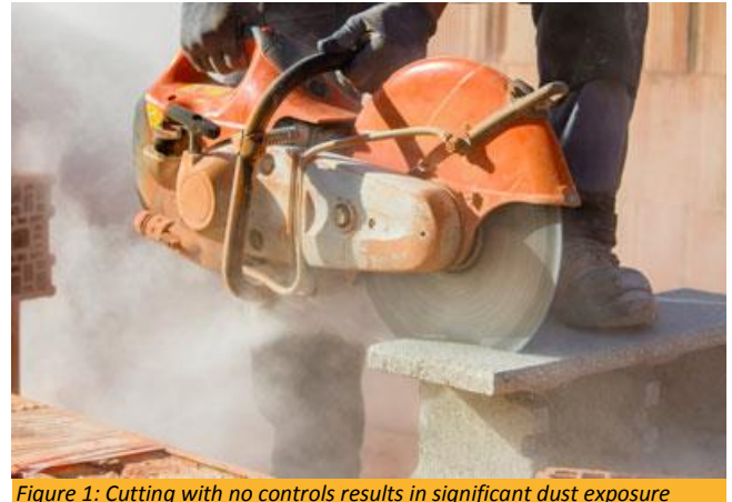
Figure 1: Cutting with no controls results in significant dust exposure
