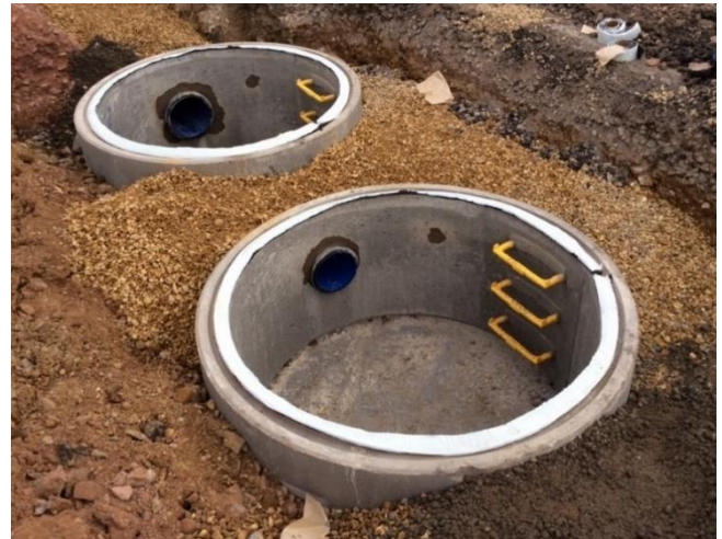
Figure 3: Using pre-fabricated chambers eliminates the need for cutting and therefore eliminates dust exposure
